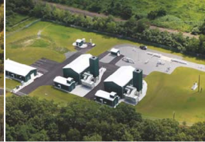
Milford, CT Compressor Station
